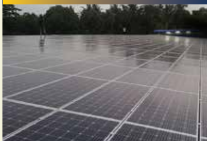
MAWATHAGAMA FOUNDATION 400KW
